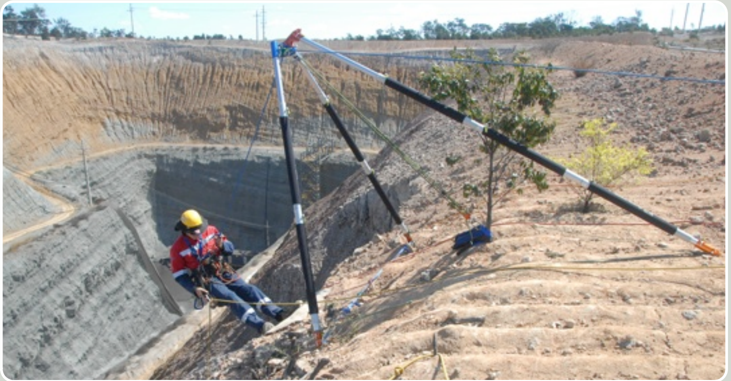
Above: Access and retrieval system for strata repair work on Carborough Downs mine highwall.
