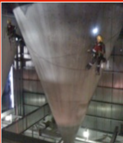
Above: Ultrasonic thickness measurements of the lower cone section of a coal storage bin
