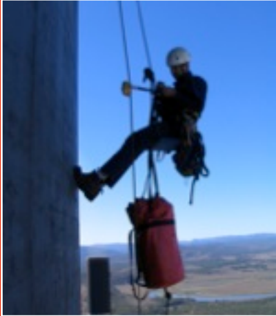
Above: Visual inspections of chlorinated rubber coating on the 220m level of a chimney wind shield
